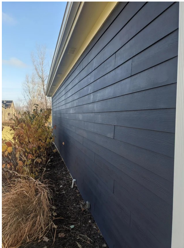
Flashing on painted vinyl siding. Lighter, patchy bands interrupt the appearance of the dark finish.
